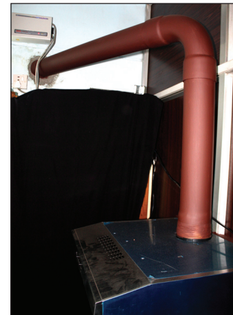
Figure 3: The outlet of the smoke evacuator (chimney) routed out of the operating room through the overhead outlet
